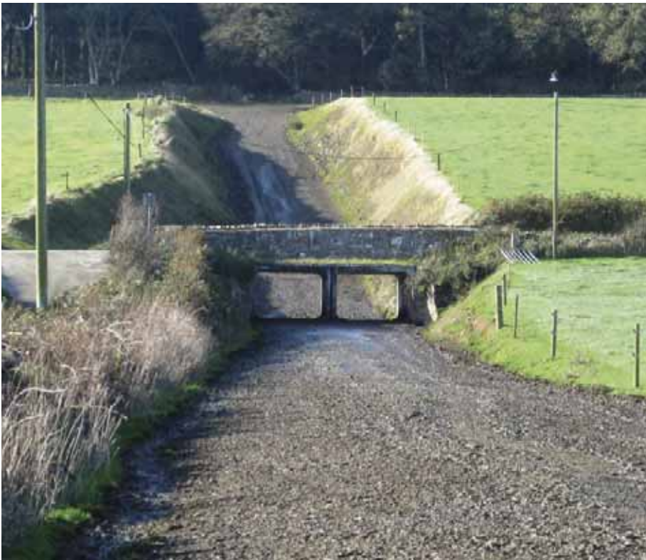
Underpasses are a big investment but can give access to grazing that would otherwise be cut off by public roads
